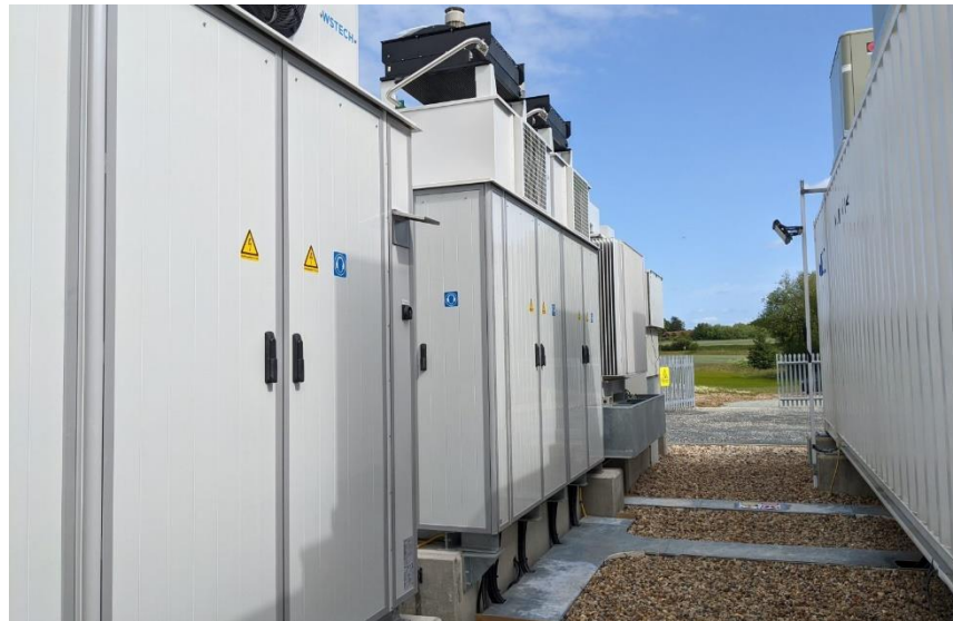
Oxfordshire County Council - £1m battery storage
