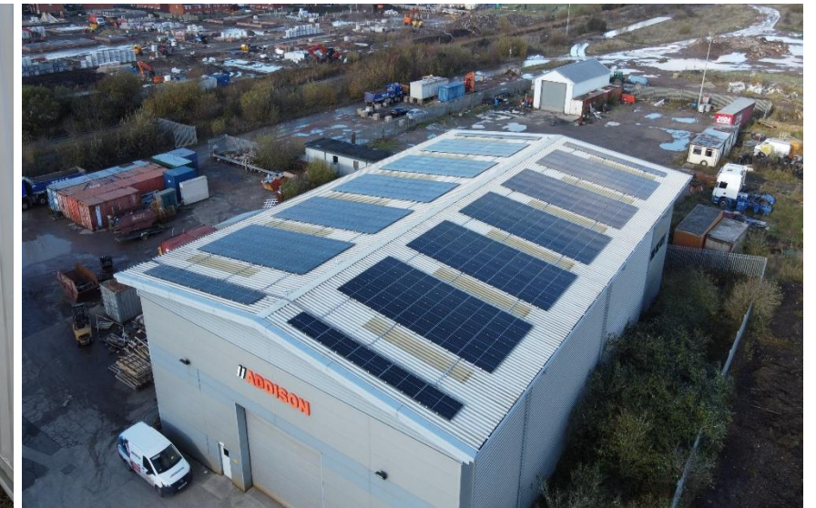
Addison Engineering 87 kWp
